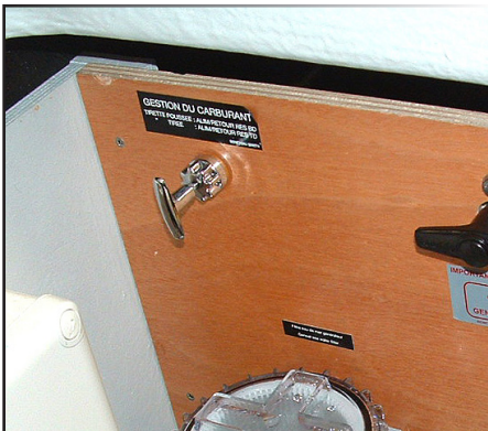
TANK / GENERATOR SELECTION PULL ROD
