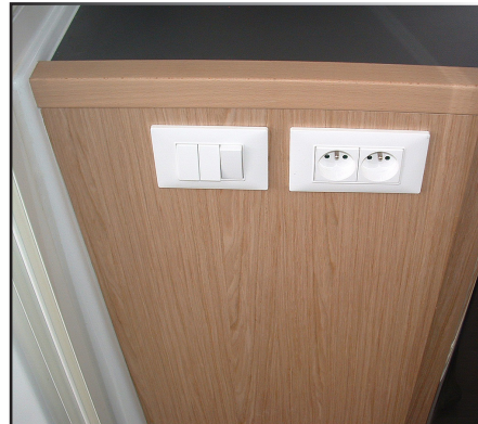
LIGHTING SWITCHES + ENTRANCE ELECTRICAL SOCKETS
