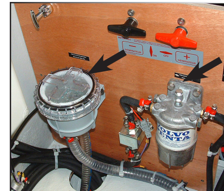
WATER FILTER + FUEL FILTER OF THE GENERATOR
