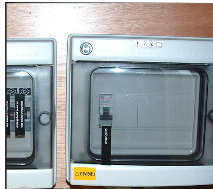
AUTOMATIC BREAKERS OF THE GENERATOR
