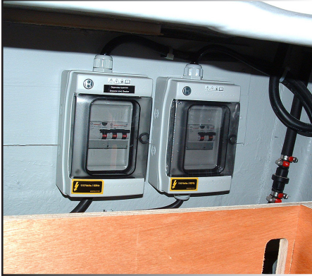
AUTOMATIC BREAKER OF A SHORE POWER SOCKET
